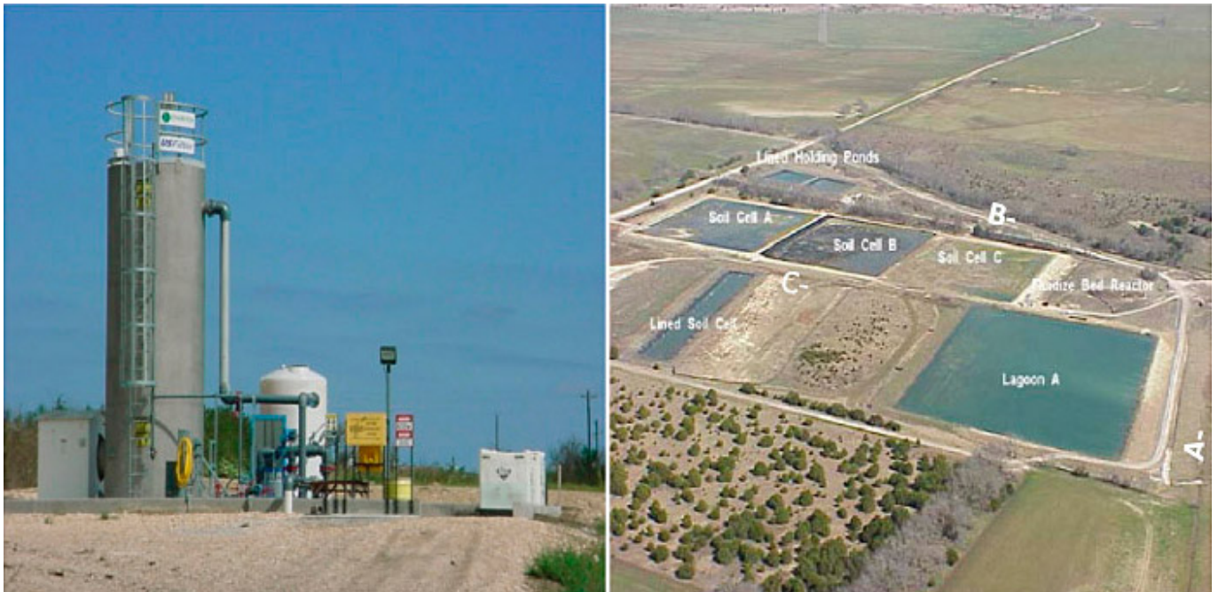
Figure 62. Fluidized bed reactor (FBR) on the left and treatment system components and water management system on the right (NAVFAC SE, 2016).
